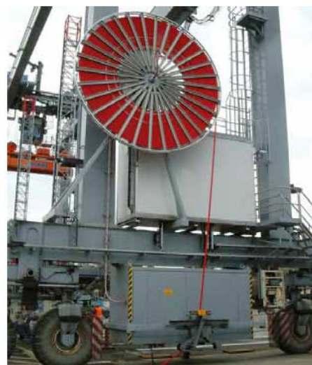
Motor cable reel in RTG operation
